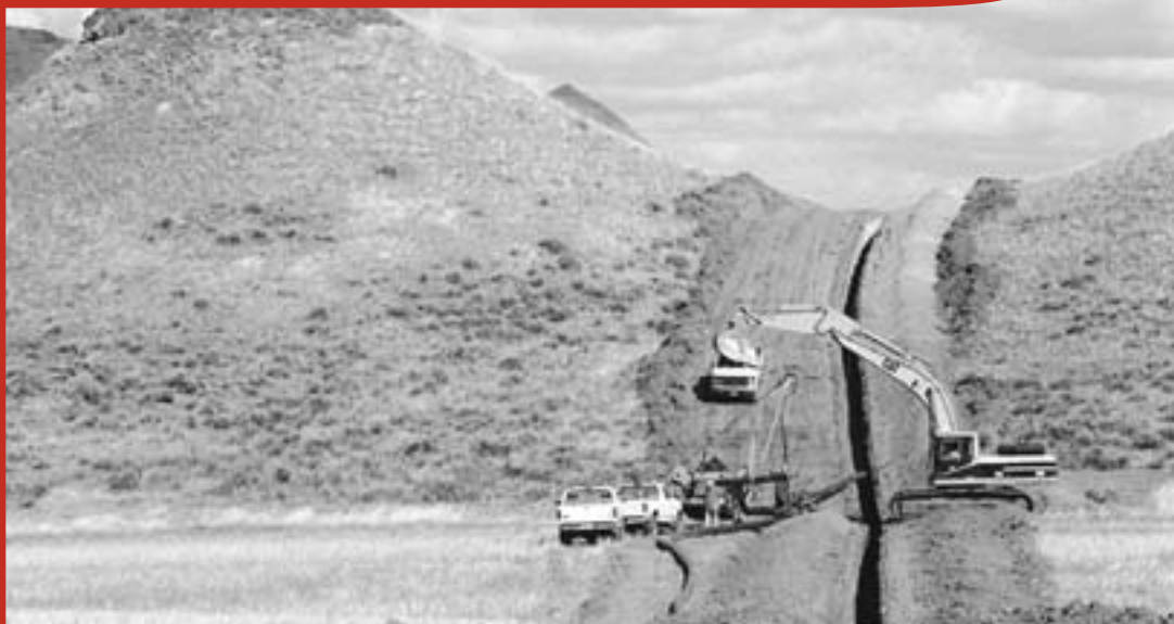
SCARS: Energy workers dig a trench for gas and water pipelines on the Sorenson family homestead in the Powder River Basin (Kevin Moloney photo)
