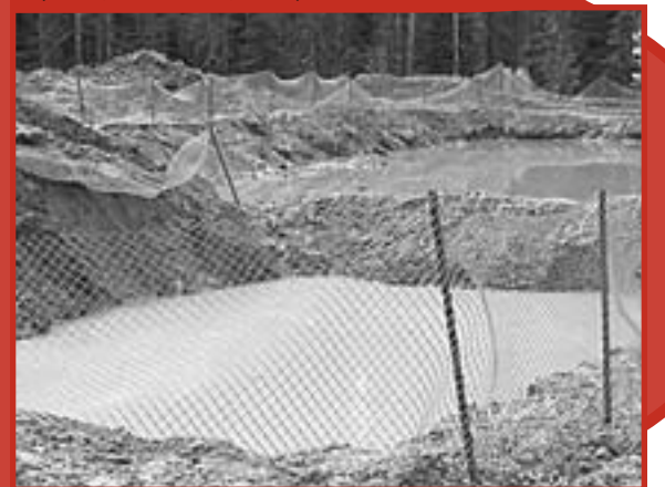
Tumbledown fencing fails to separate people and wildlife from Shell Canada’s open, unlined waste pit for coalbed methane drill waste (Casey Brennan photo)
